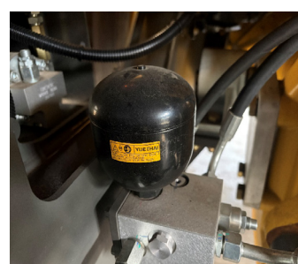
Line Burst Valve
